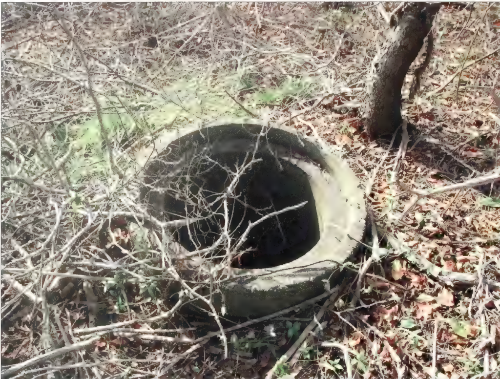
Figure 5.93. Concrete pipe on southern slope of Battery Mills. The concrete pipe should be capped to prevent possible injury and reduce water entering into or around the underground structures (Olmsted Center, January 2009).
